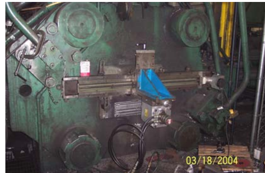
On-site milling of Extrusion press
