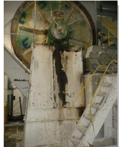
Ball mill with concrete pedestal
